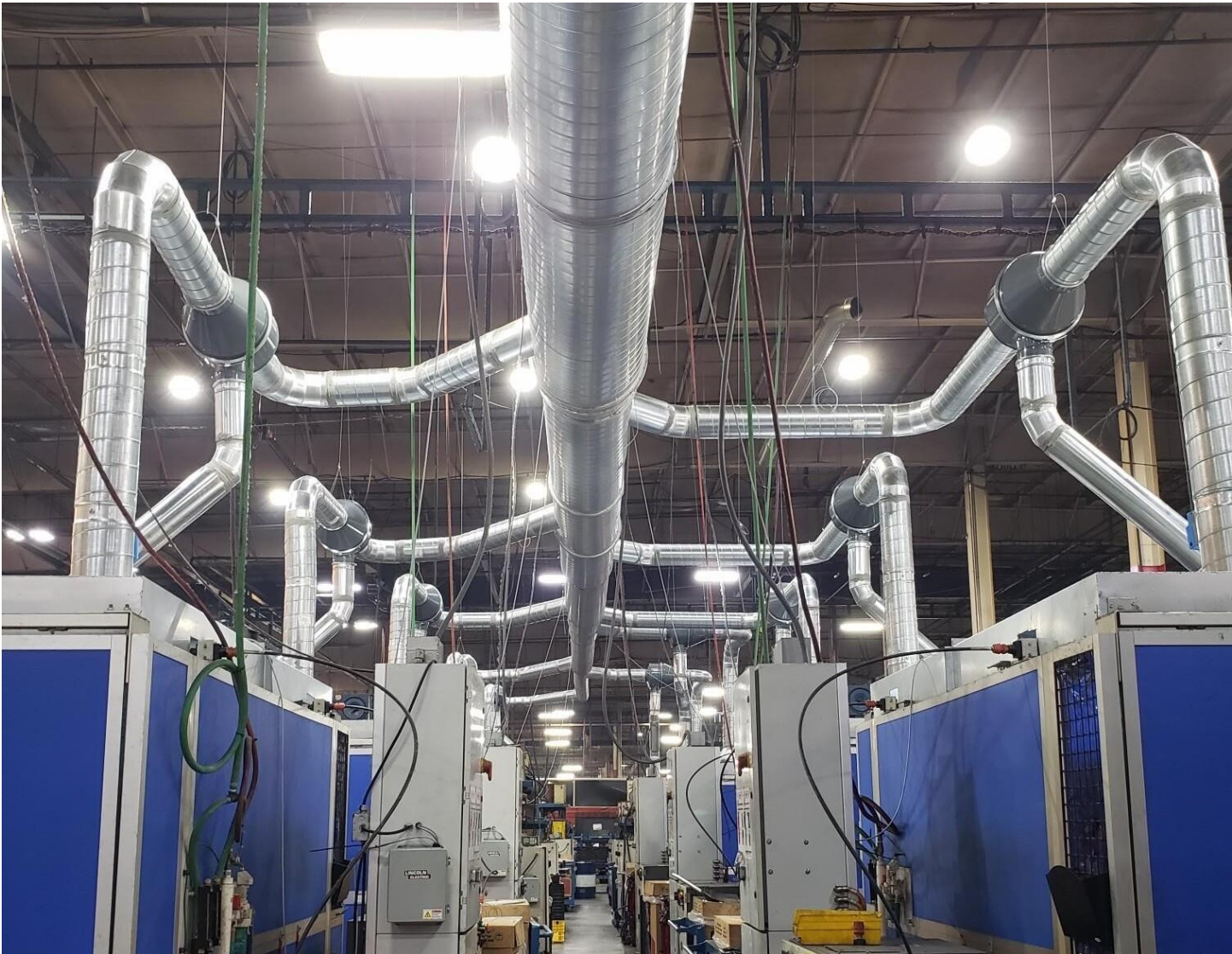
This features Dust Duct installed in a manufacturing plant in Ohio.
